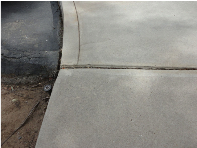
47. Trip hazard in concrete sidewalk
