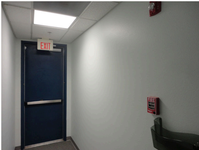
23. Exit sign in corridor
