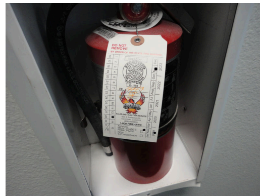
Current tag on fire extinguisher
