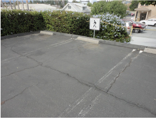
Cracks and faded striping
