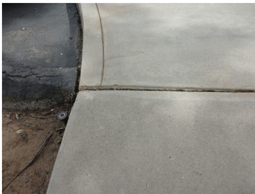
Trip hazard in concrete sidewalk
