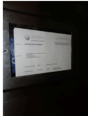
28. Expired elevator tag
