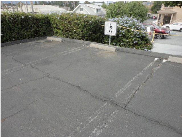
7. Cracks and faded striping
