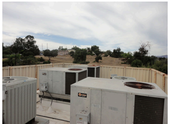
40. HVAC units on roof
