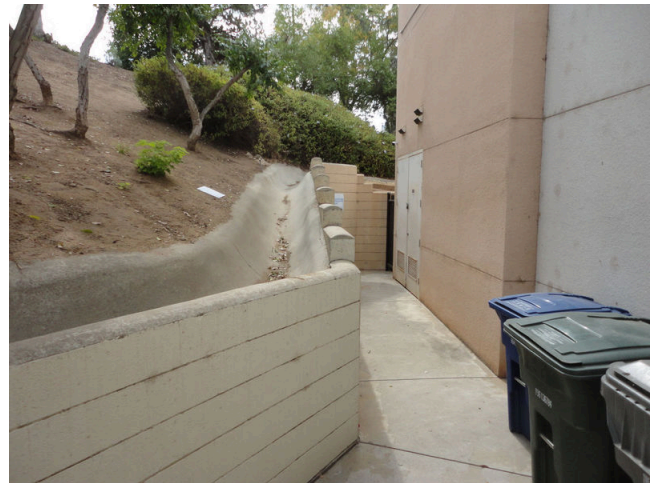
50. Area of water intrusion into elevator pit
