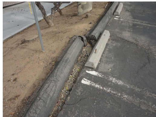
Broken asphalt curb
