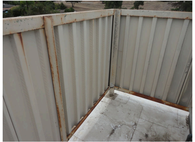
42. Rust on metal screen on roof
