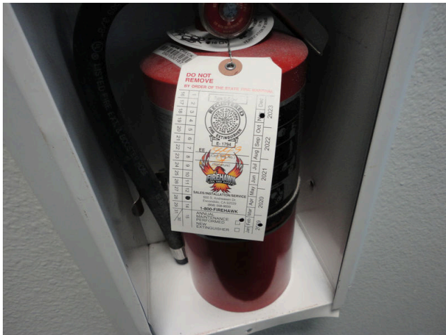
35. Current tag on fire extinguisher
