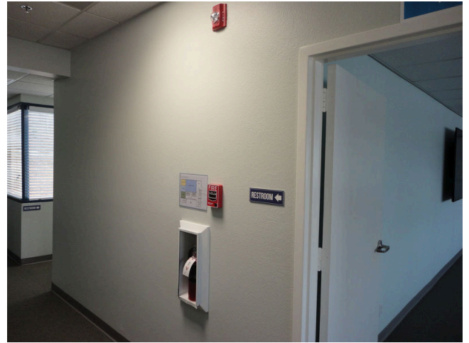
34. Fire extinguisher alarm and pull box
