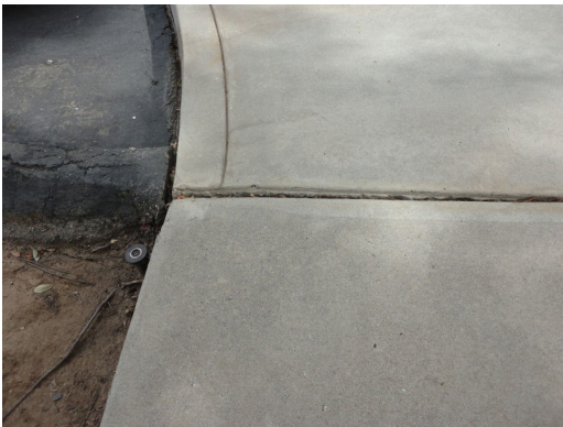
Trip hazard in concrete sidewalk
