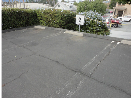
Cracks and faded striping
