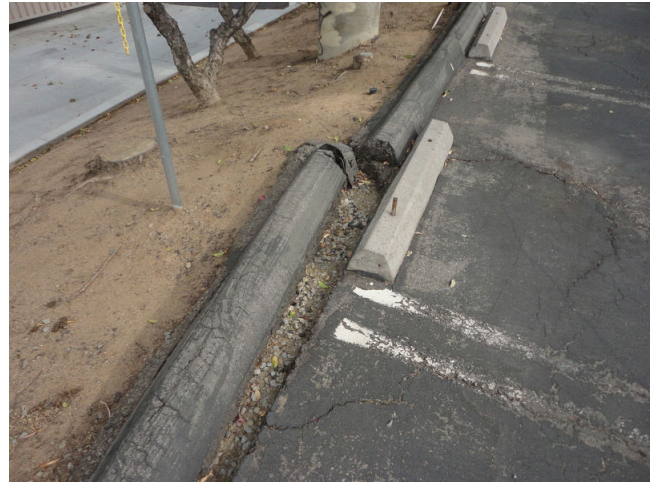
46. Broken asphalt curb
