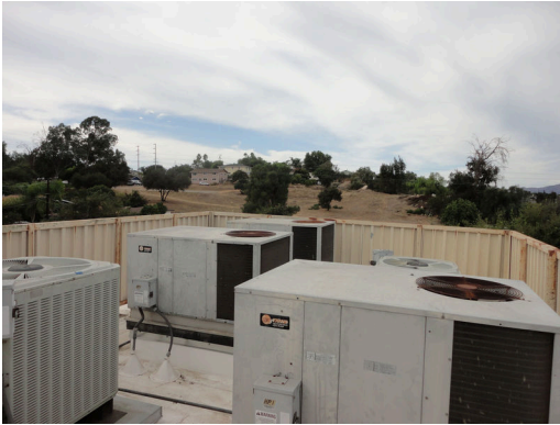
HVAC units on roof
