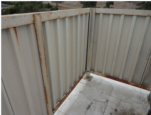
Rust on metal screen on roof
