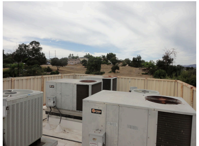
40. HVAC units on roof
