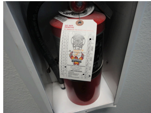
Current tag on fire extinguisher
