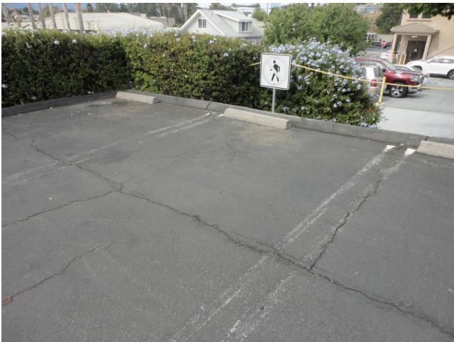
7. Cracks and faded striping
