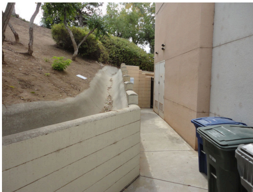
Area of water intrusion into elevator pit
