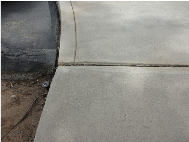
47. Trip hazard in concrete sidewalk
