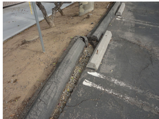
Broken asphalt curb
