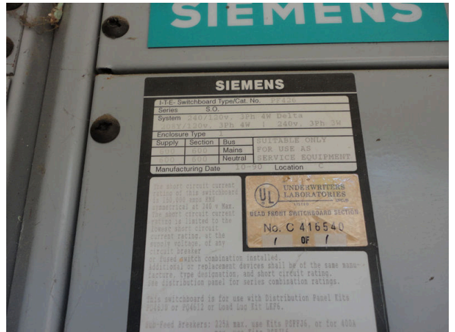
44. Service rated at 600 amps
