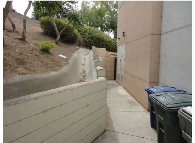
50. Area of water intrusion into elevator pit
